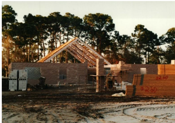
Block walls up and nave arches in place on new construction site.
